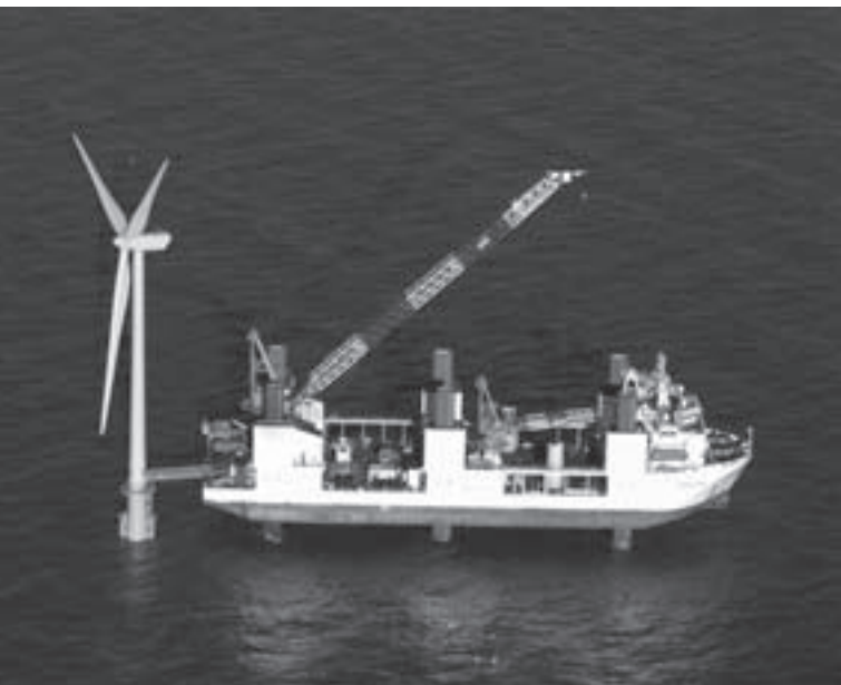
Barrow wind farm, UK
